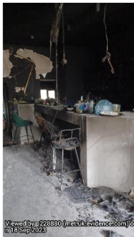
Exhibit SM/2 – Picture of inside Monak (facing towards the rear of the premises)
